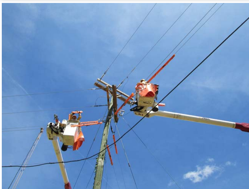
CVEC crew in East District relocating a pole on a 3-phase line.
